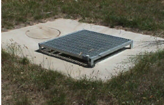
Figure 24.4 Grated Sump Field Inlet
